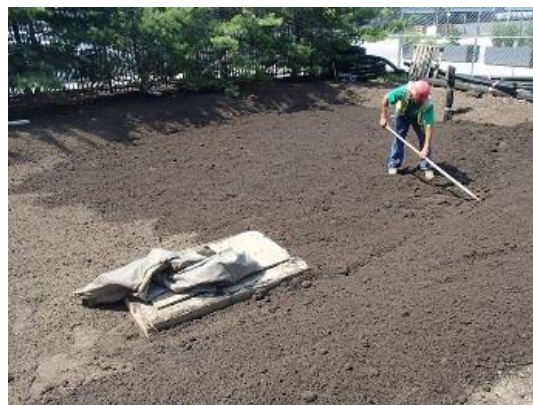
An example of a bioinfiltration basin installation
